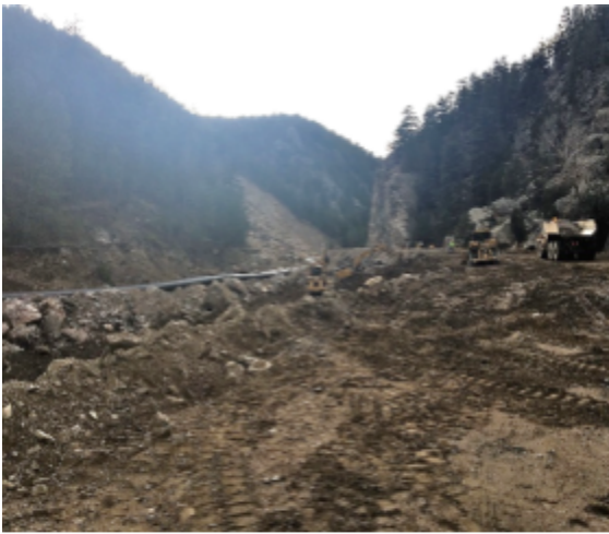
Photo 17.3 Construction of a matrix riprap revetment along the Big Thompson River on US 34, Larimer County, Colorado, near MP 72.
