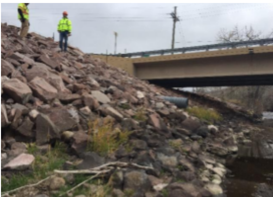
Photo 17.1 Rock riprap treatment along US 287 on the bank of the Cache la Poudre River in Larimer County, Colorado.
